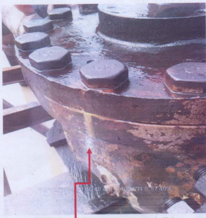
Fig B: Incident facility (insulating joint)/ leak point
