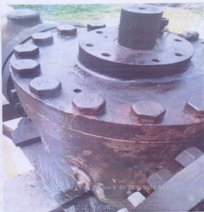
Fig C: Incident facility after tightening of the loose bolts
